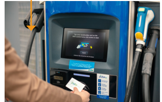
Charging point reader
